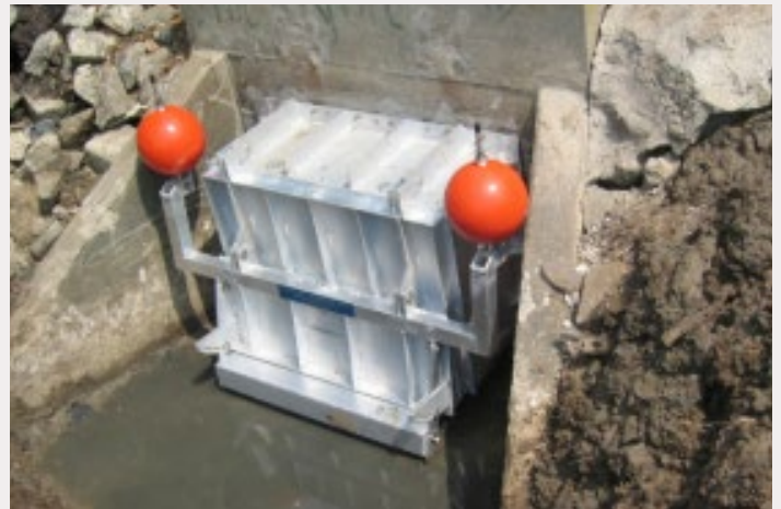
Tide gate enables water flow into the reserve ( http://www.goldenharvestinc.com/ )
