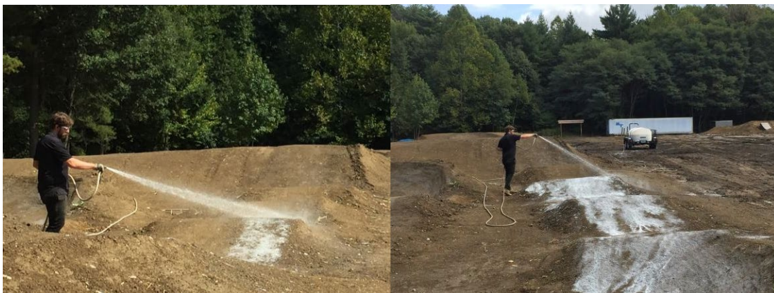
Applying soil stabilizer at the beginning of the season to extend the functional life of a pump track.
