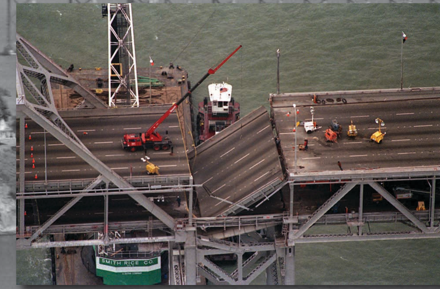
Damage from the 1989 Loma Prieta Earthquake.
